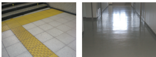
Rugged walkway surface
